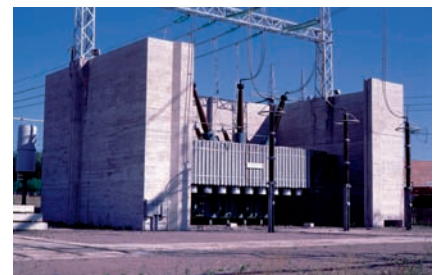
The determination of moisture in oil is an essential part of a comprehensive transformer maintenance program.
